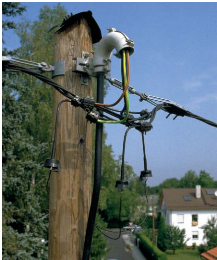
Transition: insulated overhead lines to cables
